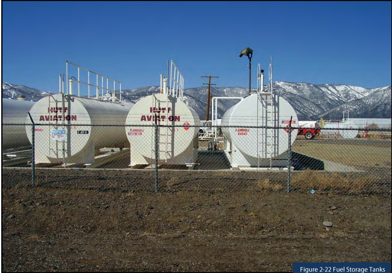
Figure 2-22 Fuel Storage Tanks
